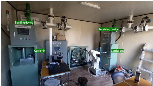
Fig. 6 Pneumatic tube main system
