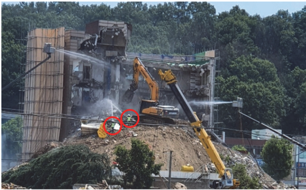
(a) Manual water spraying in a demolition site [5] (Adapted from Ref. 5 on the basis of webpage)
