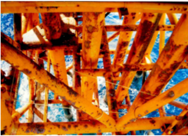
Fig. 1 Platform BK-1 at White Tiger field was corroded (photo by VSP)
