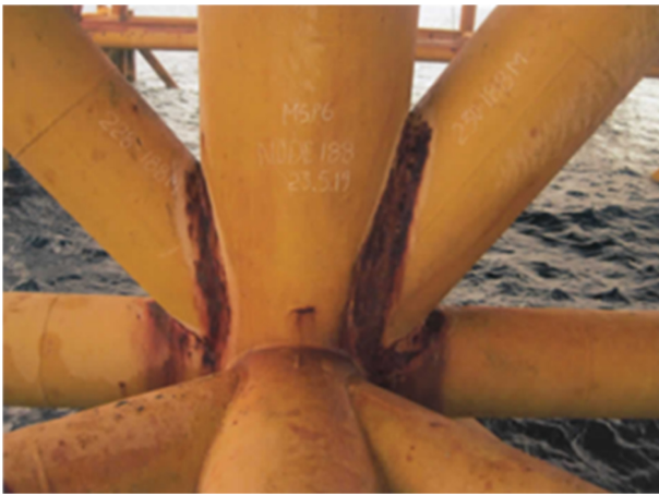
Fig. 2 A tubular joint in the platform MSP6 at White Tiger field was corroded (photo by VSP)
