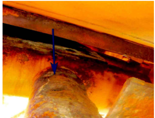
Fig. 3 A tubular joint in the platform MSP6 was corroded (photo by VSP)
